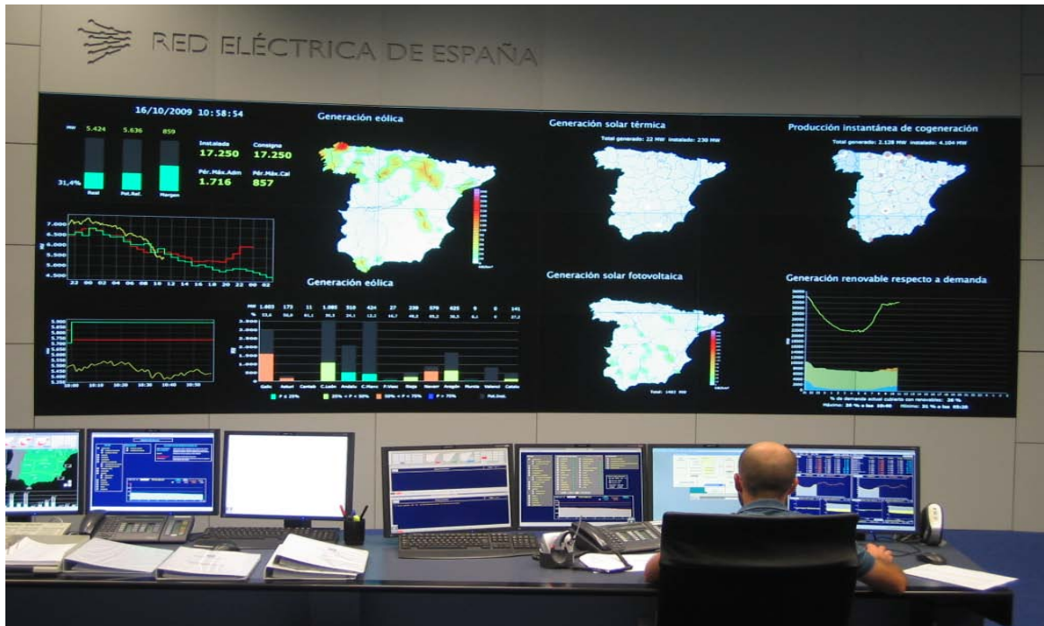
Figure 86. General View of the Control Center for Renewable Energy, CECRE (Provided by Miguel de la Torre, REE)
