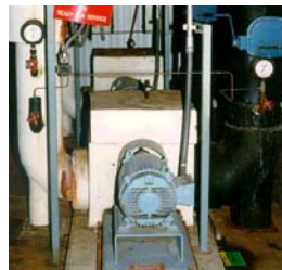
Pump head: 36 m Flow rate: 97.6 m 3 /h => hydraulic power: 9.6 kW Combined pump and motor efficiency = 59%
