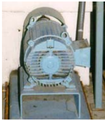
15 kW Motor Efficiency is ~ 91%
