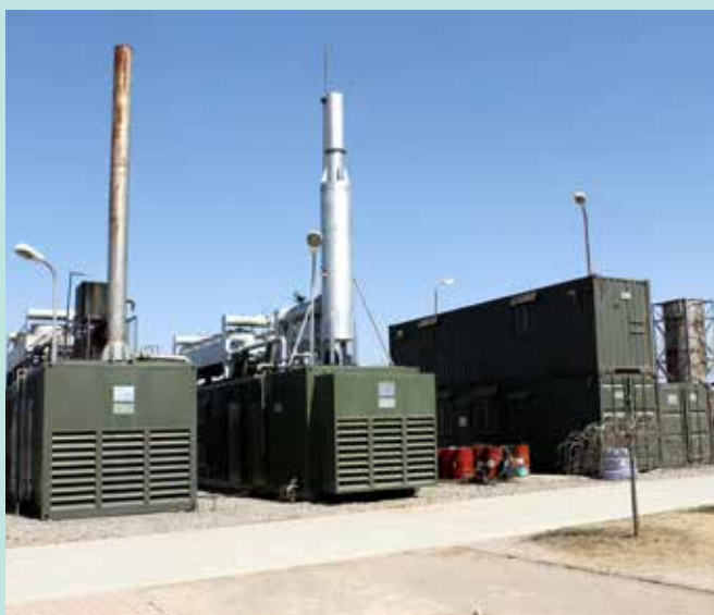
A power generator that uses captured landfill gas in China. (Credit: Yang Aijun/WorldBank)
