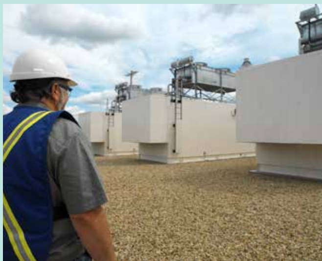
Electricity generators use landfill gas as fuel in Edmonton, Canada. (Credit: Pembina Institute)
