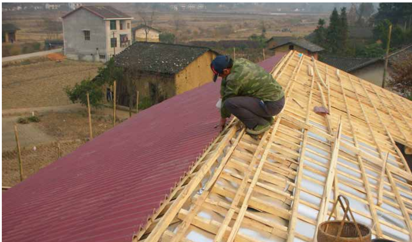
A double layer aluminum roof improves the “thermal envelope” of a house in Hunan Province, China helps to reduce heating requirements. (Credit: He Jianqing)
