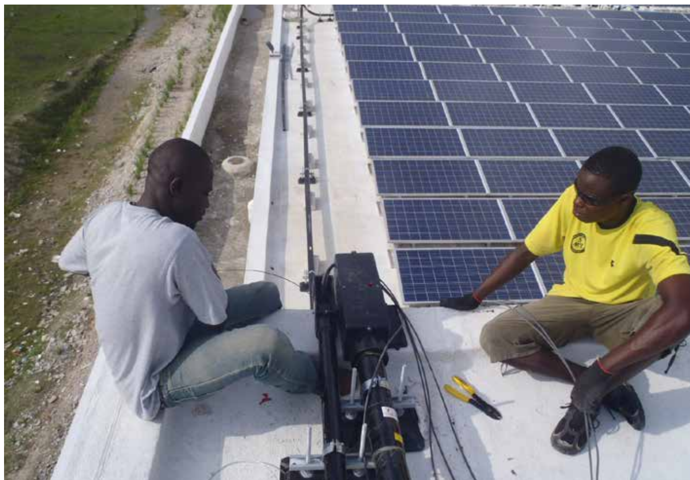
Construction workers adjust equipment for the photovoltaic solar power system on the roof of University Hospital Mirebalais, Haiti. (Credit: Jon Chew/Partners in Health)
