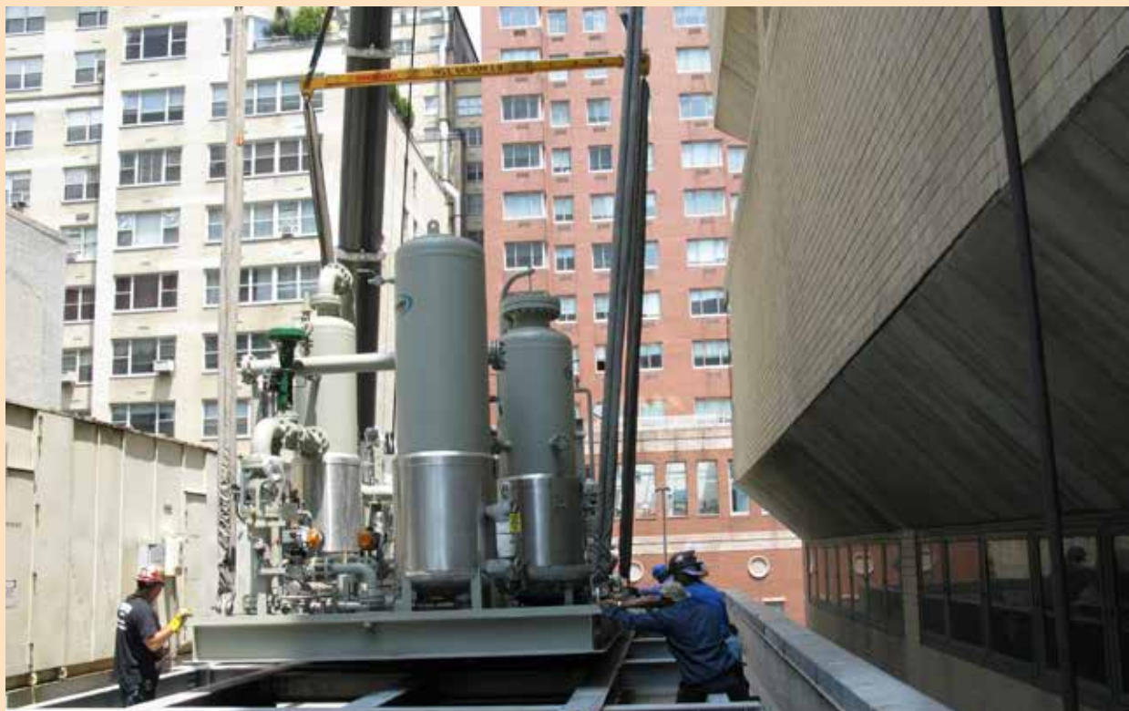
Gas compressor installed as part of New York-Presbyterian Hospital’s Combined Heat and Power system. (Credit: New York-Presbyterian Hospital)
